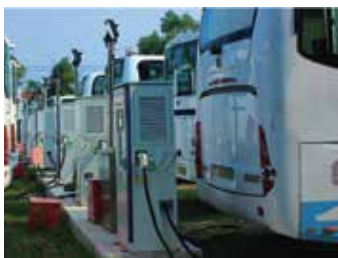
Shanghai Longdong Avenue Charging Station
