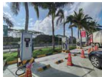
Hainan Sinopec Gas Station Service Area
