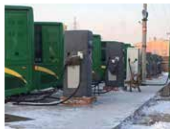
Harbin Bus Charging Station
