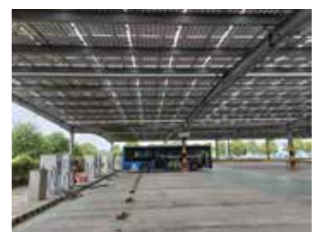
ZhenJiang Photovoltaic-Energy storage-Charging Station
